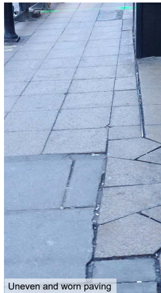
Uneven and worn paving
